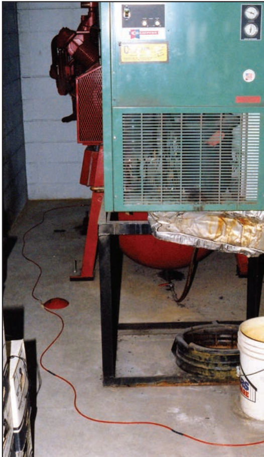
Water Alert / Sensor Cable in mechanical Room
