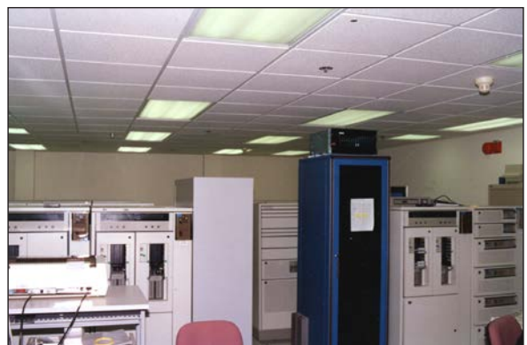
View of 1500 sq. ft. computer room after Ceiling Guard installed.
